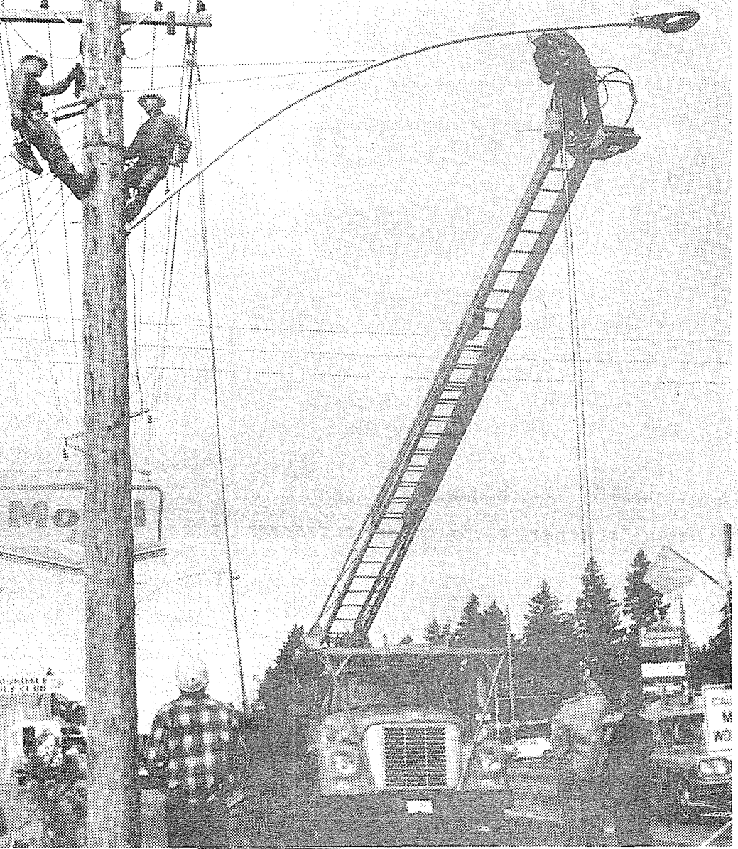
INSTALLATION of mercury vapor street lighting along Pacific Avenue between 131st and 152nd started Monday, October 17. Completion of the project is expected within the next two weeks. Elmhurst Mutual Power and Light Company officials said Monday. Pending availability of twenty foot extension arms lighting will eventually be installed to 168th and Pacific.
