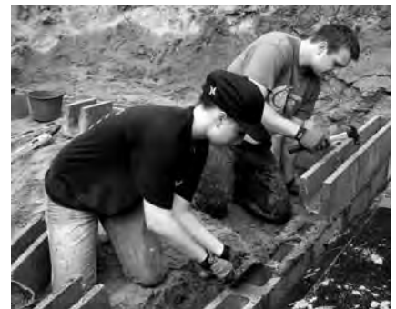
Nichole and Tyler Kurz begin to lay the foundation that will be the home of a Guatemalan family.
