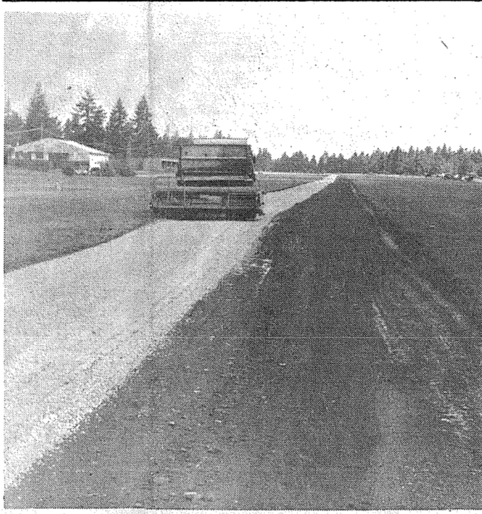
THE SPANAWAY AIRPORT was closed for a few days this past week while crews put down a hard surface for the 2,400 foot runway. Shown above, a truck moves down the runway towing a spreader. 'Slim' Lawson, popular proprietor, says the runway improvement will add to the comfort and safety of the flying public. —Times Journal Photo
