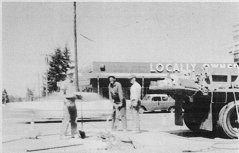
FREAK HAPPENING — A section of Pacific Avenue, at the Bargain Basket Grocery Store, broke loose Monday and created an obstacle of 5 inches of concrete for northbound drivers to overcome. Officials stated that the moisture underneath the road combined with the recent heatwave caused the near dilemma. County construction workers soon had the situation under control.
