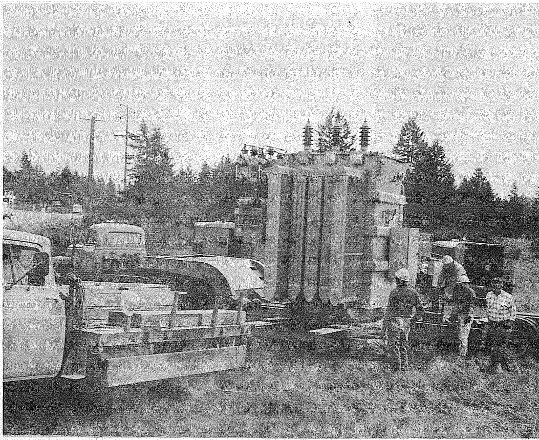
HELPING HAND —A 52,000 lb. transformer is moved into position by Tacoma City Light for temporary help to Elmhurst Mutual while a substitution is overhauled. The transformer has a capacity of 2500 KVA at 50,000 volts.
