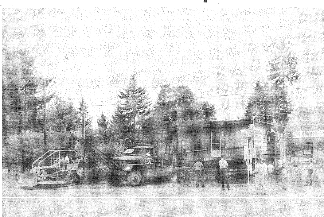
MOVING DAY — Ready for the expansion of South End Hardware's building at 185th and Pacific, house movers prepare to take the house on the north side of the building off the lot. Bill and Dorothy Righetti, in announcing their plans to expand, reaffirmed their faith in the growth of the South End and stated that their plans were going ahead for an expanded building.
