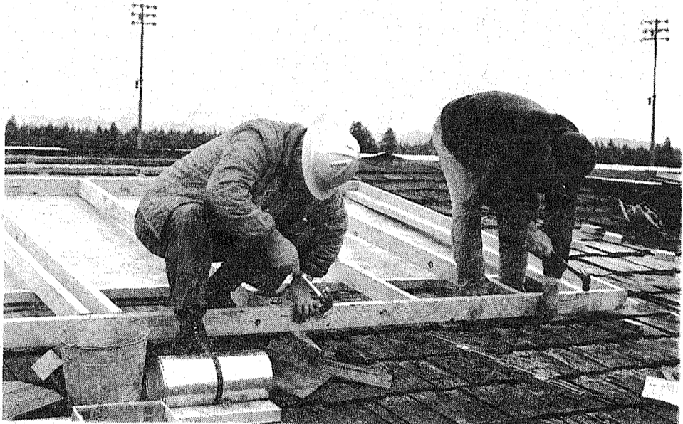
WITH MT. RAINIER providing the background, workers prepare frame for new press box. Completed structure will seat public address announcer, scoreboard operator, and statisticians. (Upper) Two by Fours are cut to size on roof of grandstand. About 15 Bethel Boosters turned out for work party.
