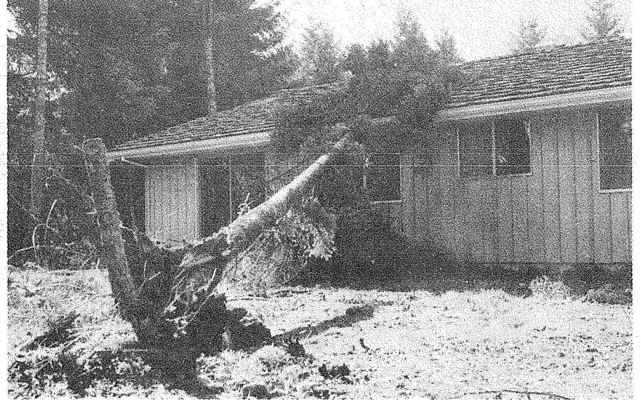
STORM VICTIM. This 60 foot fir yielded to a windstorm Friday night and crashed into an unoccupied house on 43rd Avenue East Near Shady Acres Airport. The structure was recently completed and has not yet been sold. Estimate of damage was not available. Note weak root system protecting tree against North winds.
