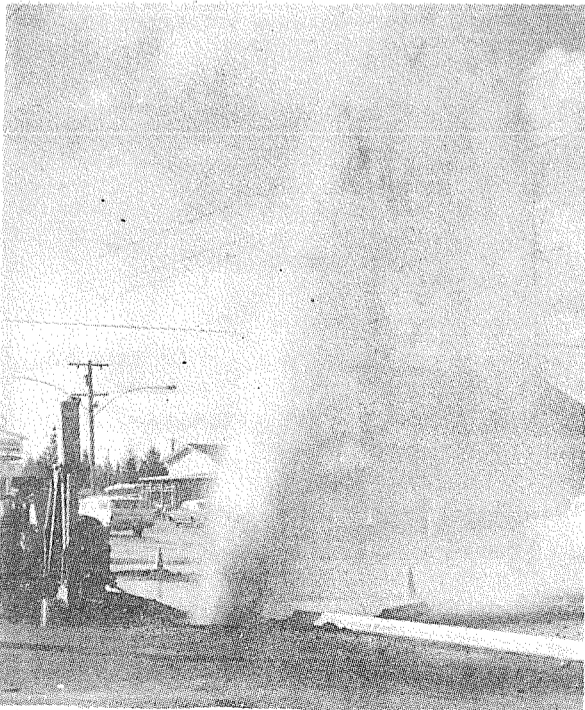
BROKEN MAIN at 136th and Pacific Ave. March 17 resembled Old Faithful. The 6 inch main carrying water at a 85-90 pounds pressure was punctured accidentally by construction workers and showered Pacific Avenue with rocks and water.
