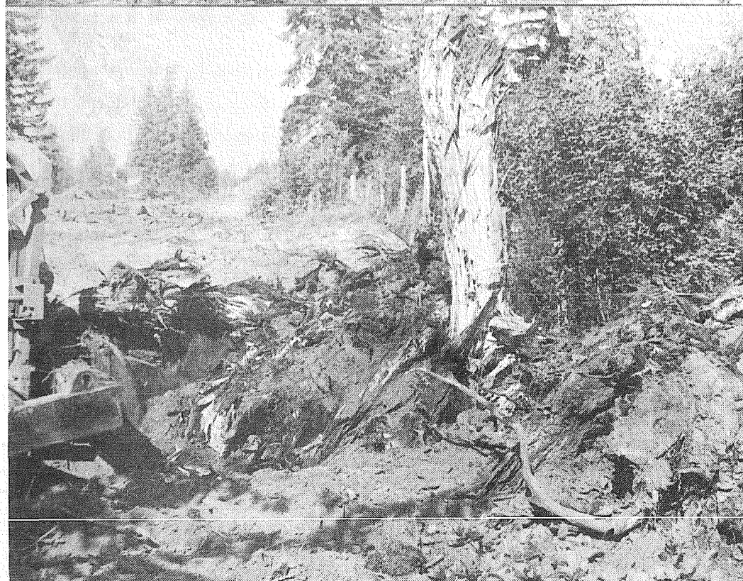
FAST WORK — George Wallen, Eatonville, operates the big tractor demolishing stumps as clearing work on the addition to Highway 5-G began last week. In the top photo, a side view of the stump-breaker is shown. In the second photo the splitter aims right at the camera through a stump on the rightofway. The splitter completes its devastation of a one-time tree in the third photo, and in the bottom photo, Wallen backs off the tractor to await clean up of the shattered stump. The whole operation takes about 5 minutes. —Times Journal Photos
