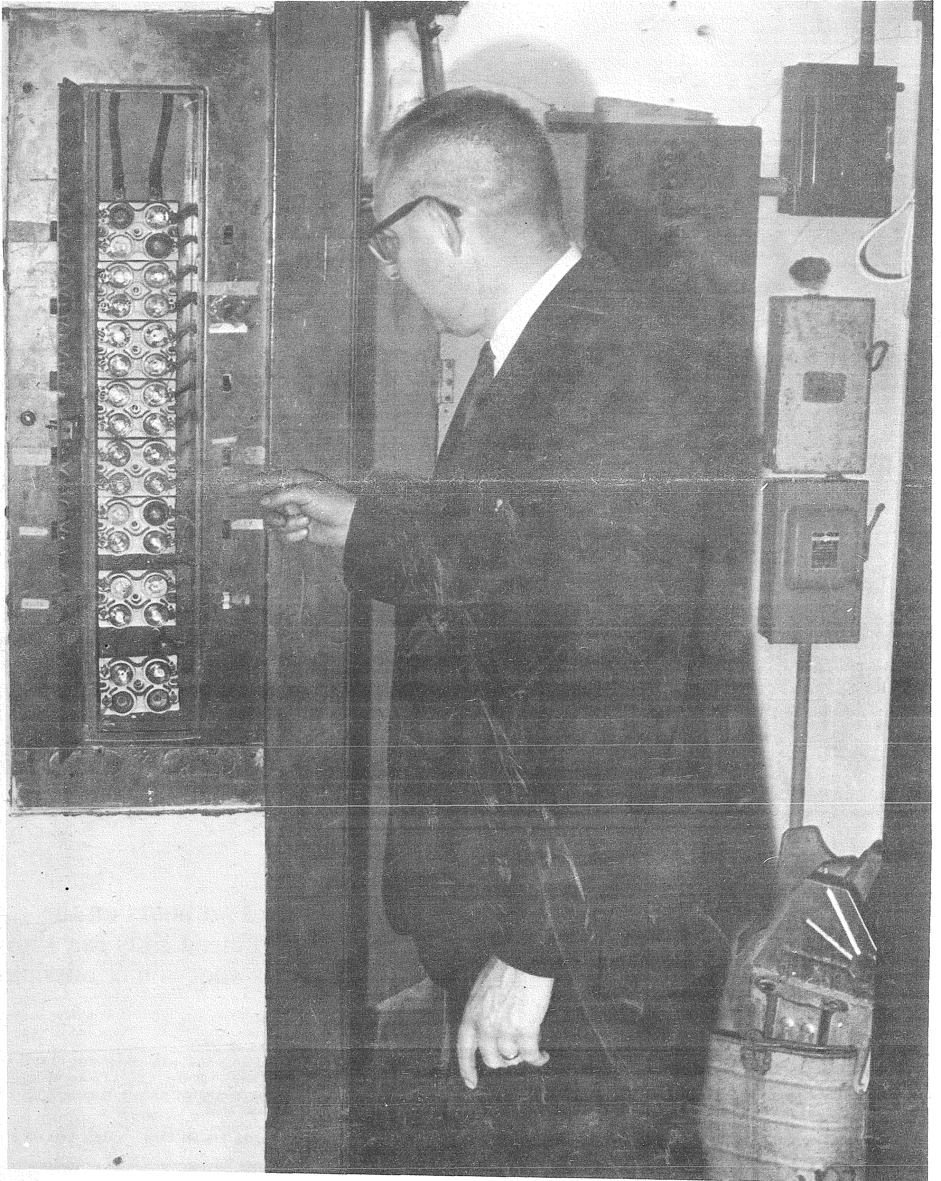
EARL SOLIE, Spanaway Elementary School principal, points to outdated master fuse box servicing brick building of Spanaway School complex. Wiring throughout
