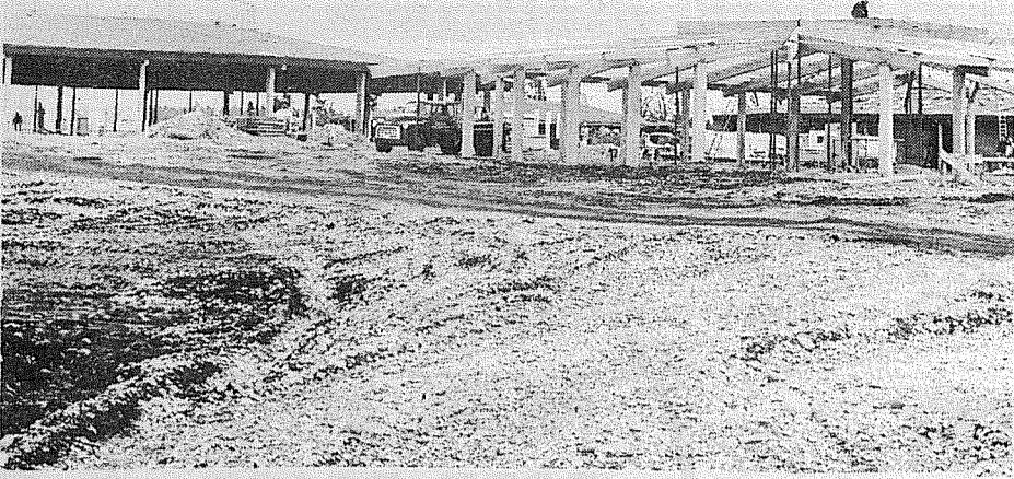
WASHINGTON HIGH SCHOOL begins to take shape as workmen prepare to roof another of the pavilion-like structures. The new high school for the Franklin Pierce District, at the intersection of Tule Lake Road and Spanaway Loop Road features several of the circular buildings for maximum flexibility. Scheduled to open in the fall the new facility will house a thousand students.
