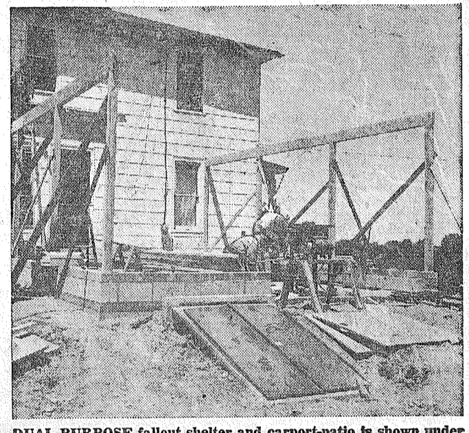
DUAL PURPOSE fallout shelter and carport-patio is shown under construction at the farm of John Holden near Hickory Corners, Mich. The shelter, to be used also for food storage, cost $1,200. With the carport and patio now being added, the cost totaled $2,300. Holden's family of three, and eight neighbors, gave the shelter a realistic workout recently when a small tornado struck nearby. An entrance to the shelter is in the foreground. (OCDM Photo)
