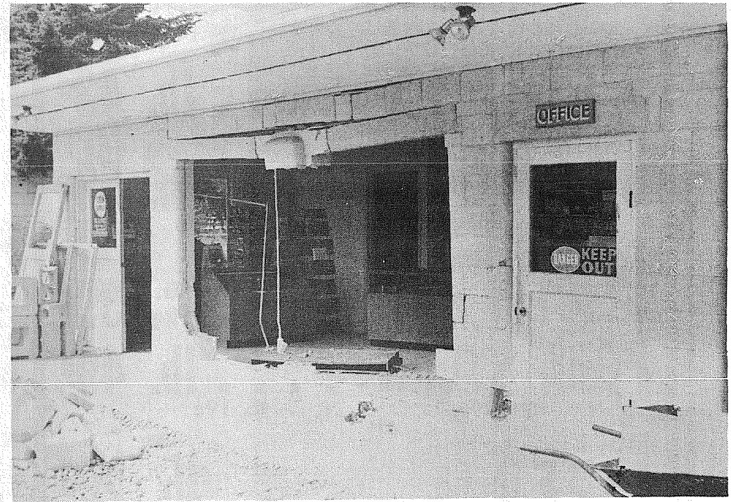
UNWELCOME VISITOR — An early morning visitor made a new entrance in the Blauvelt Printing Company building on Portland Avenue last week when he drove his station wagon into the front of the building. The extensive damage was being repaired this week, and business was being conducted, not quite as usual. —Times Journal Photo
