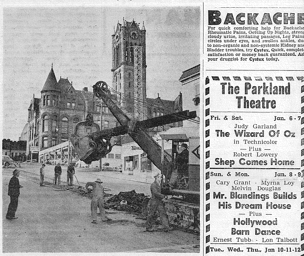
In the shadow of the shrinking courthouse tower, Abe Bergersen, former Commissioner of Public Works, directs the laying of a new power cable. Note outside hoist on courthouse used by tower wrecking crews.
