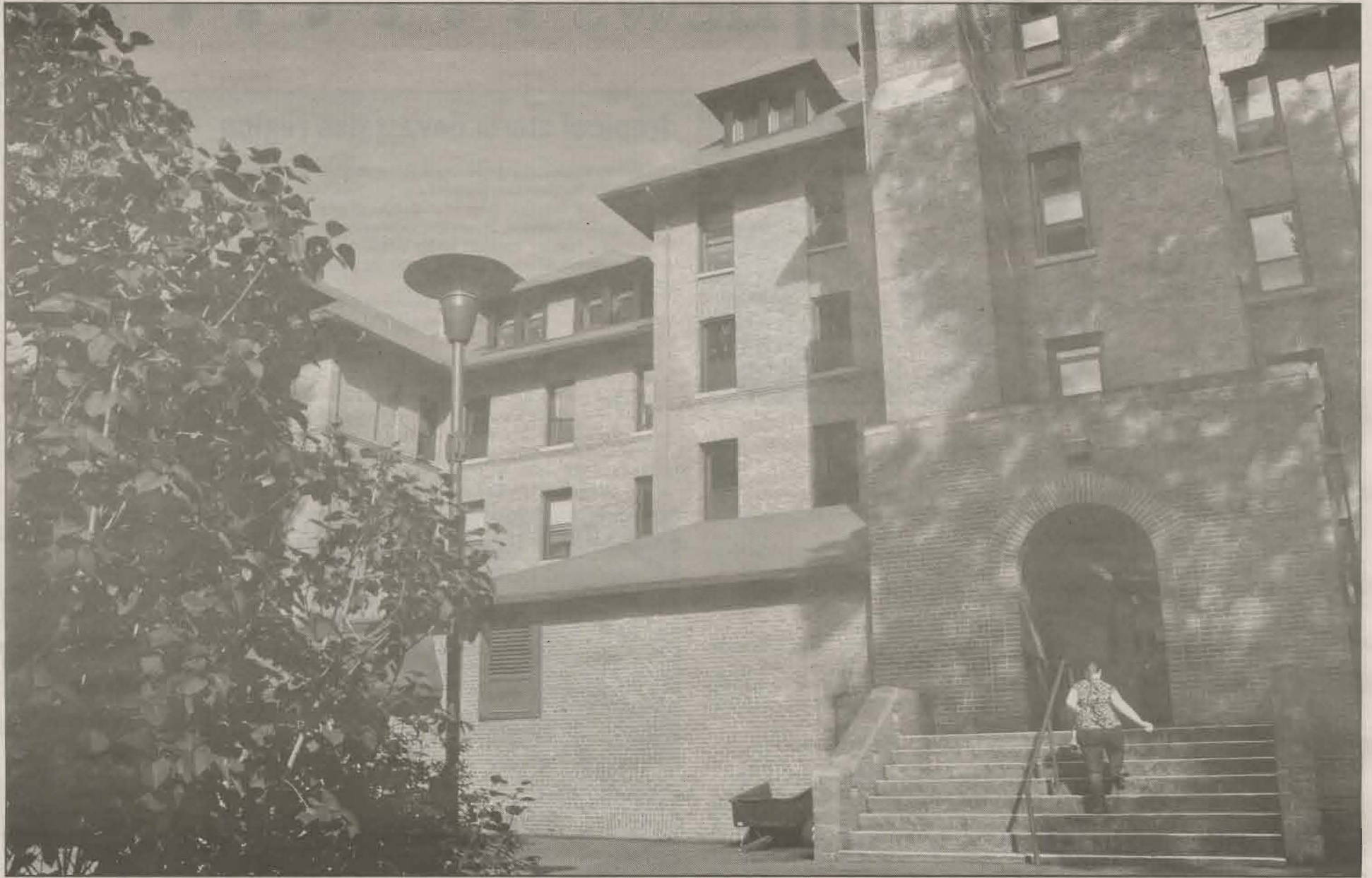
Water unexpectedly flows into Harstad as students begin to move into resident hall, wrecking rooms and causing trouble for students calling it home.
