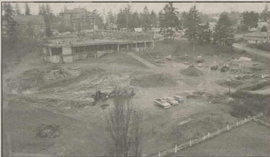
Construction on the new building in 1970 required significant alterations to fulfill the vision of a student center.
