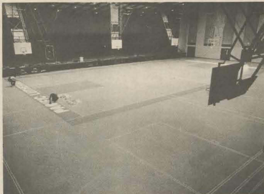
New vinyl flooring was installed in Olson Auditorium in early September. The resilient Sport Tred floor was completed in time for Opening Convocation.
