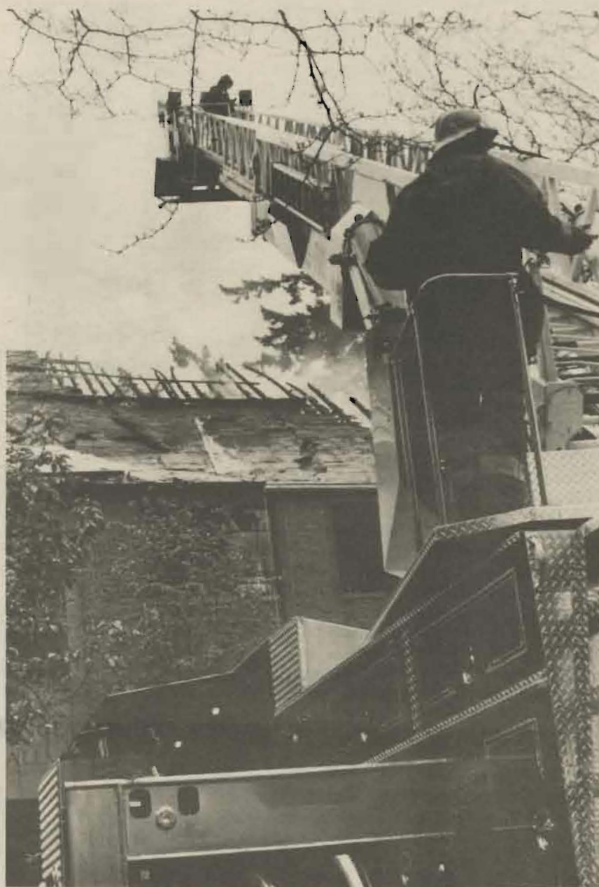
A briefly spectacular two-alarm fire in Ramstad Hall May 20 temporarily slowed renovation on the former science building. Damage was confined to areas being rebuilt, and officials anticipate that the School of Nursing and Student Life will still be able to move in in the fall.
