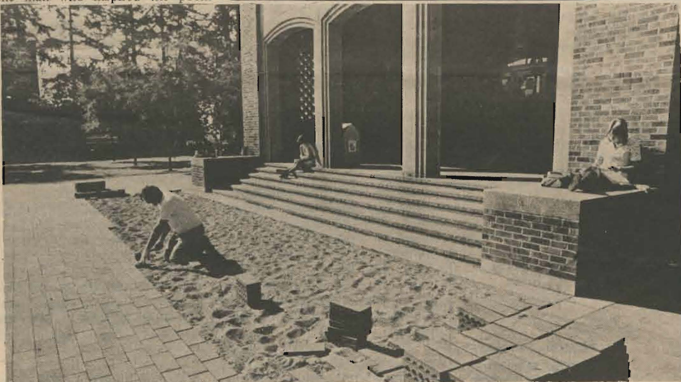
Skilled hands repair the damage done to Red Square by freshmen initiated into Ivy House. Bricks were taken from the square and stacked in front of Rainier. Ivy will have to pay for all costs, despite the fact other dorms were also involved.
