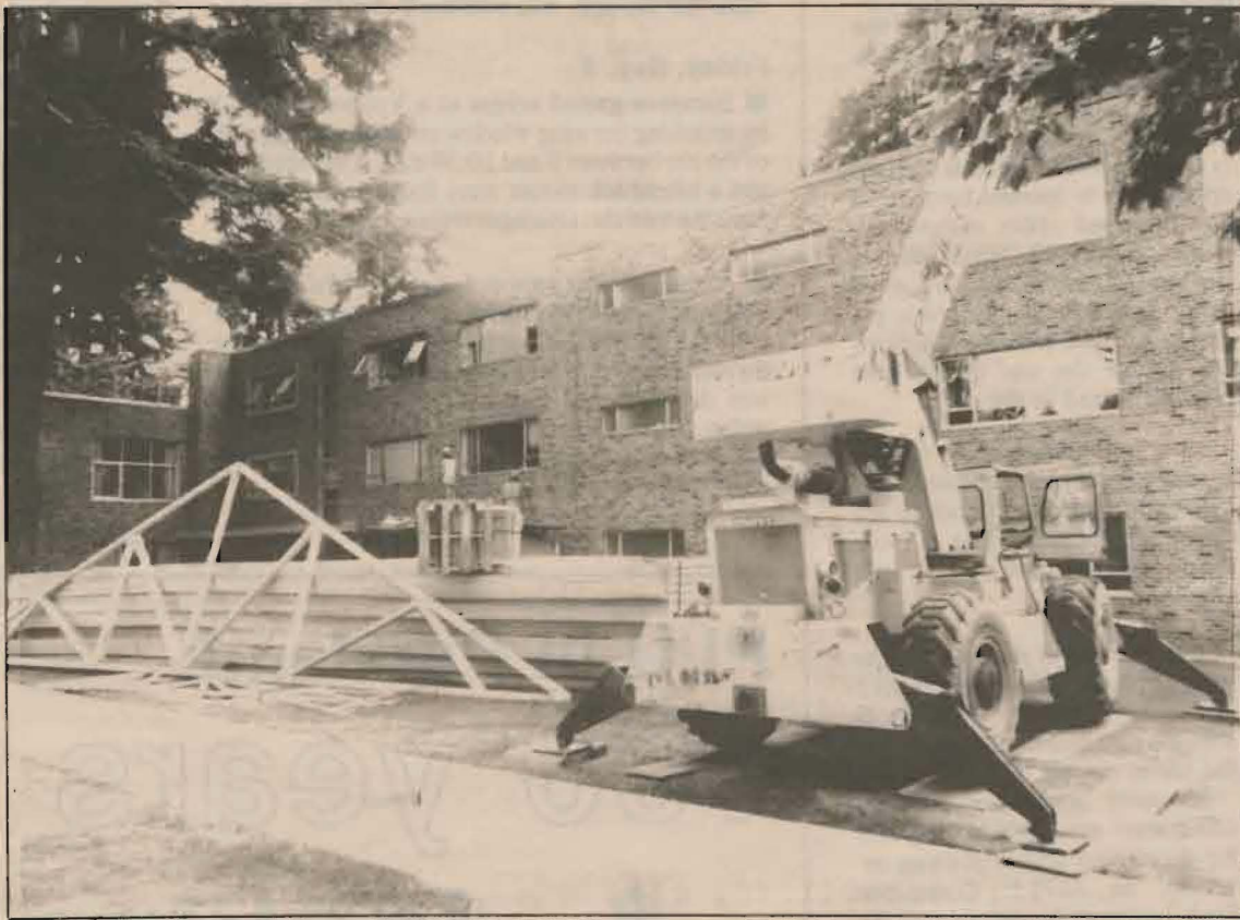
Hong hall received a needed roof over the summer months. The project cost $184,000.
