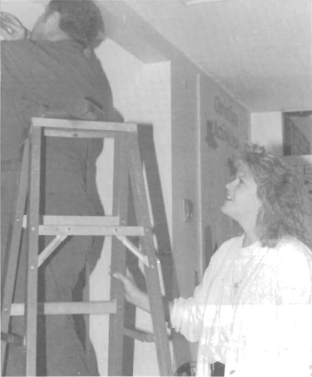
Making sure the job is done right, RA Linda Renz oversees an electrician putting in a t.v. cable in Kreidler's main lobby. (Brian Ford)
