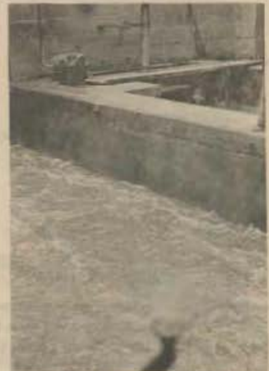
One of the many steps in treating raw sewage. Tank 4 aerates the material.
