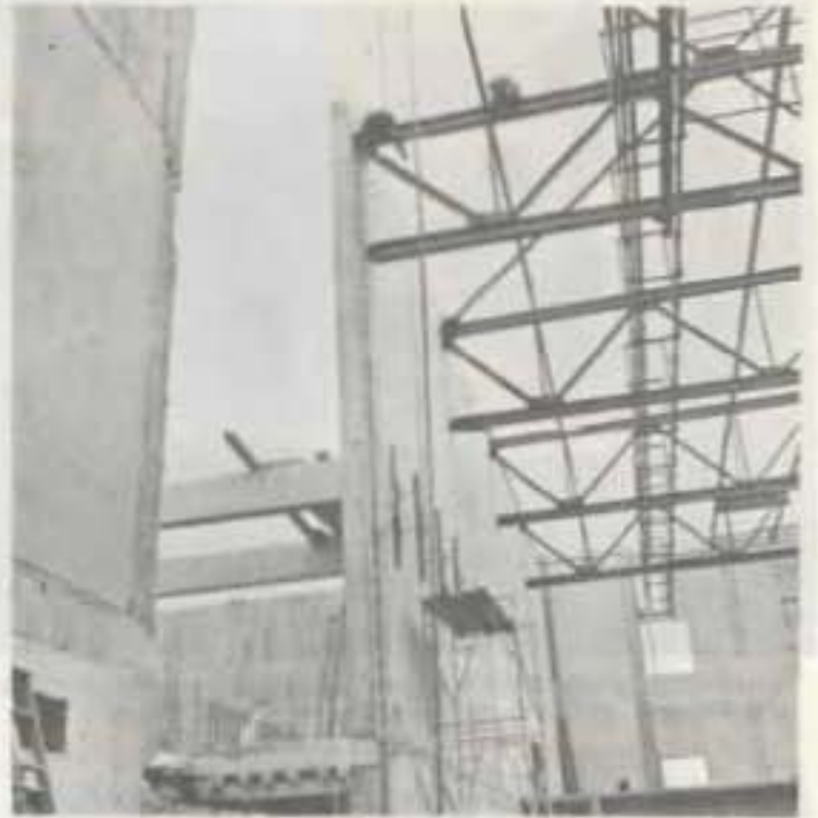
ALTHOUGH CONSTRUCTION is two weeks behind schedule, the new gym is expected to be ready for use by the beginning of spring semester.
