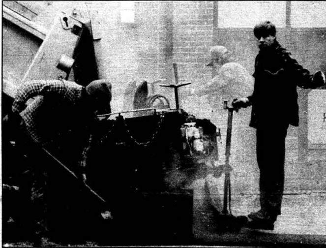
Construction posed obstacles for interim students as PLU's sewer project was completed this past month. See story on page 2.
