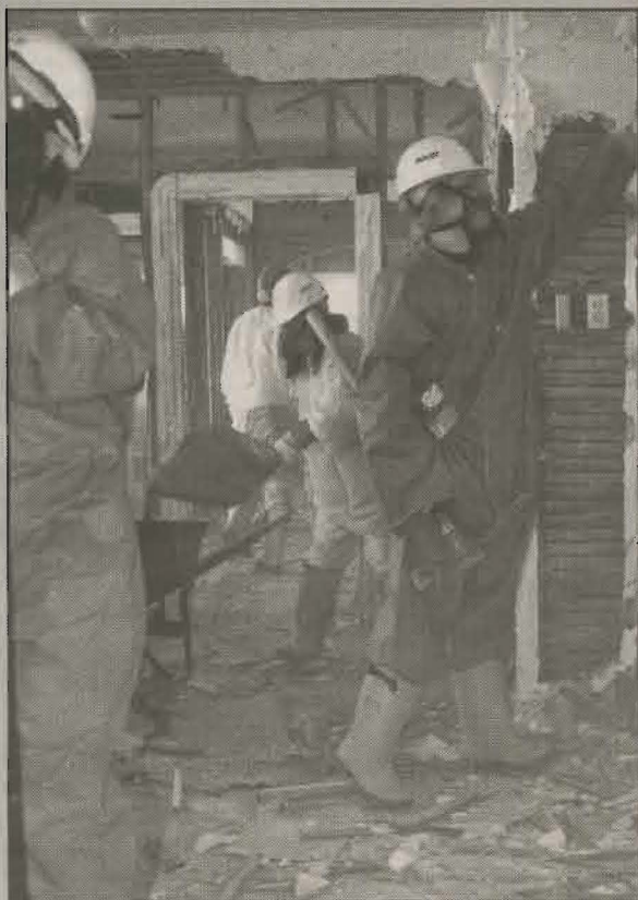
Photos courtesy of Campus Ministry PLU students gut a house in preparation for renovation. This is one of the many steps in repairing the damage cause by the hurricane
