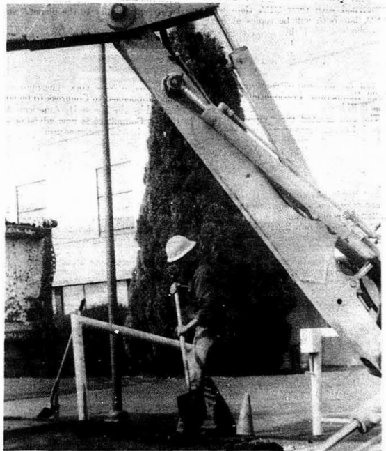
Construction winds down at the new lower campus parking lot across from Memorial Gym. The new lot should bring partial relief to the congested parking situation.
