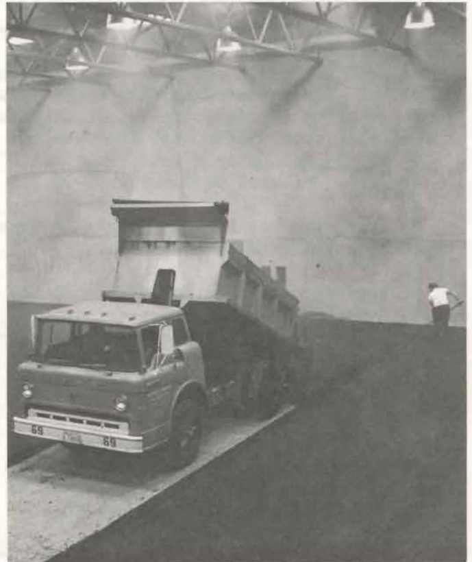
GYMNASIUM PROGRESS - Asphalt was laid this week in the new Clifford O. Olson Physical Education Auditorium Building fieldhouse in preparation for the installation of Astro-Turf next week.
