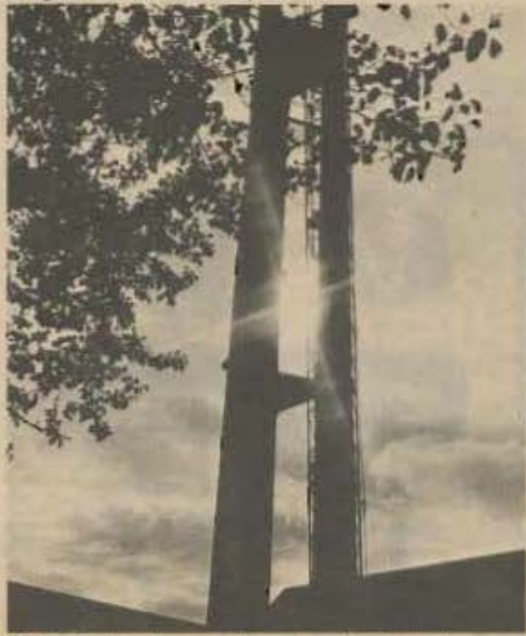
The structure of the soon to be completed clock tower looms over the University Center.
