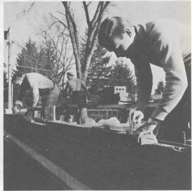
Bricklayers work toward the completion of Stuen Hall for its use in September, 1966.
