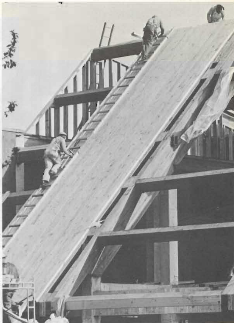
March - It's not a slide! It's the roof of the cafeteria and bookstore.
