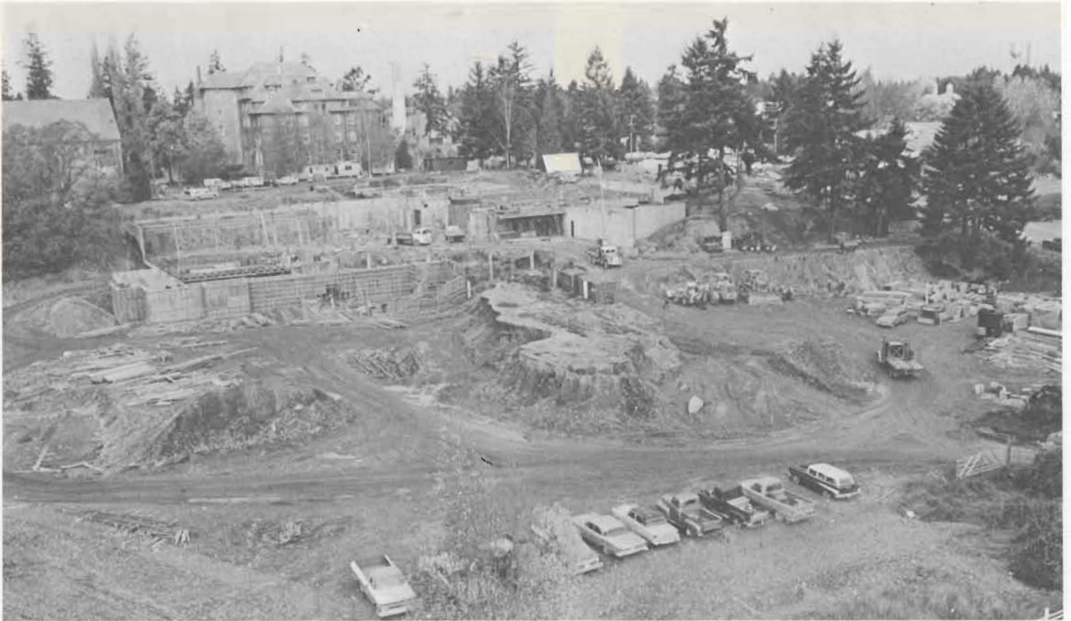
September - Excavation and foundation is well underway for the 3.2 million dollar Student Center, which is to serve as a link between upper and lower campus.
