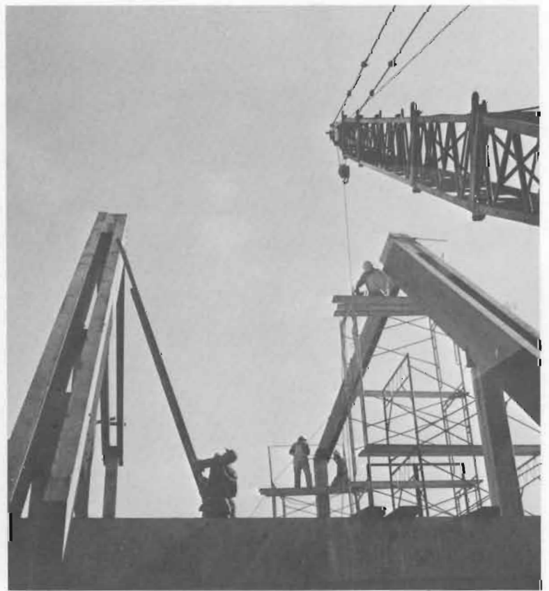
January - Workers add rafters to the University Services section on the 3rd floor.
