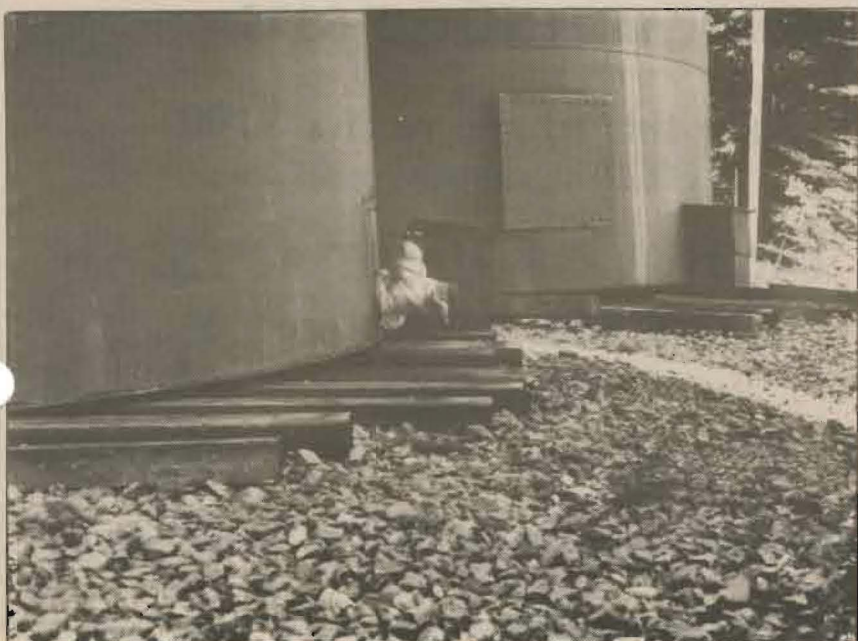
(left) "These are two 20,000 gallon water tanks, they hold the water for the community water system. One of the many geologists told Bert Johnson, who owns the land, that when the quake hit, the nearly full tanks (approximately 180,000 lbs.) jumped into the air and the ground moved four feet before the tanks landed. There are marks on the boards from where they used to sit and where they landed, without any scuff marks in between."
