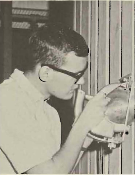
Gronberg is cutting up — the wall that is. (Remodeling the presidential suite.)
