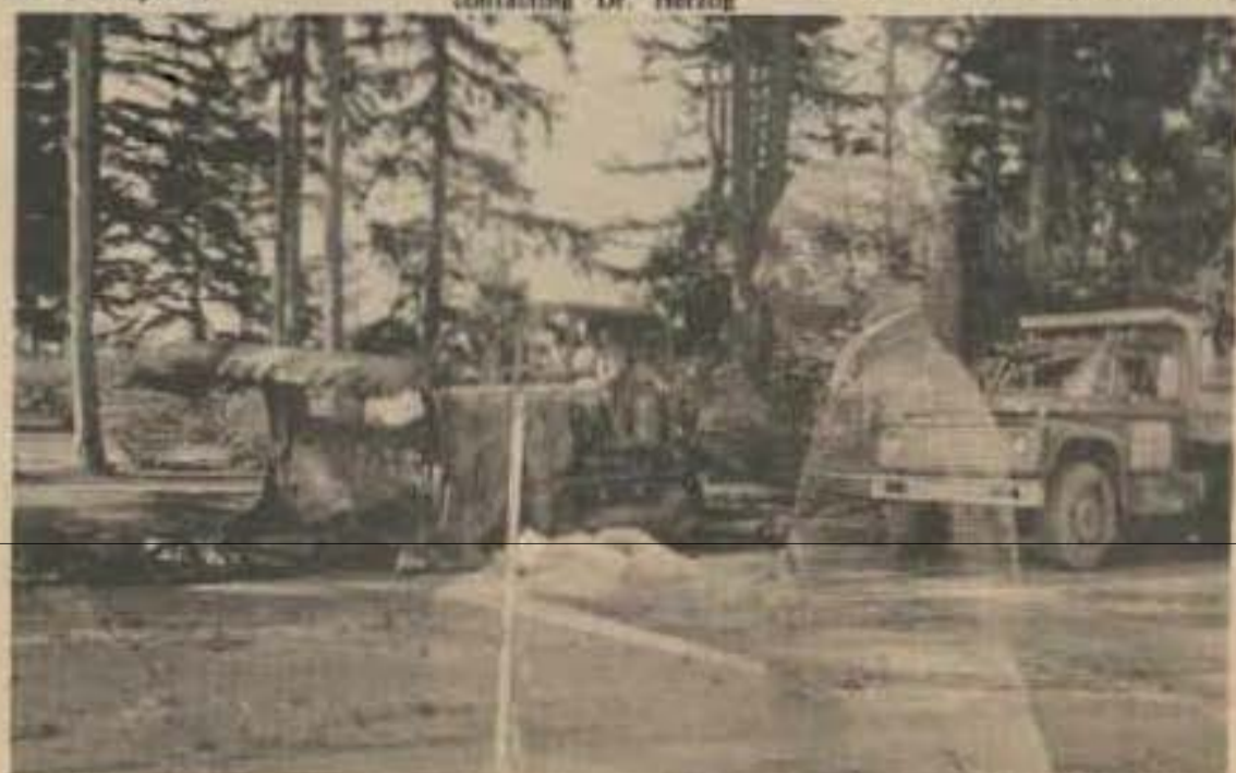
This double exposure lends a ghostly atmosphere to the groundbreaking for a new lecture hall. The building will be near the Nursing/Arts complex.
