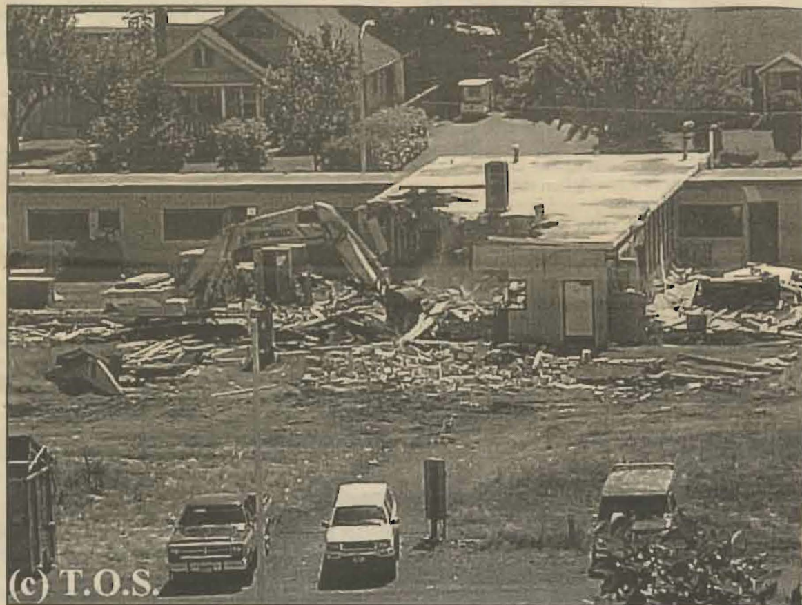
Photo by Ryan Bebe-Pelphrey A bulldozer demolishes the remains of Evergreen and Delta Courts earlier this summer.
