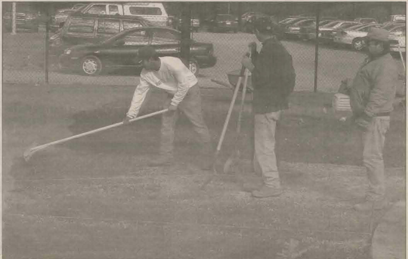
Construction workers from the Celcorp Construction Company work on a new fire access for South Hall.
