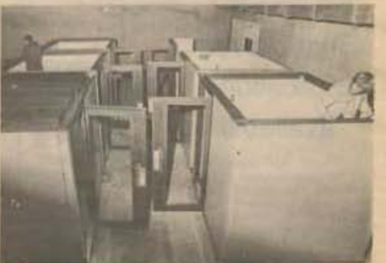
Workers are pictured erecting the new modules in the V.C. gravel pit. The modules should be ready for use next semester.
