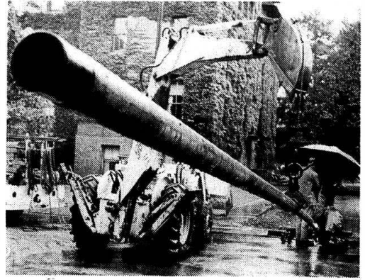
IN THEY GO —The heating system at PLU has been converted from oil to natural gas. The Washington Natural Gas Co. installed the piping this summer at no cost to the University. The annual savings in fuel cost was estimated at over $10,000 by University Business Manager Dean Buchanan. The pipe installation also involved the rerouting of several water and sewer lines to avoid having to move them later when new buildings are constructed.
