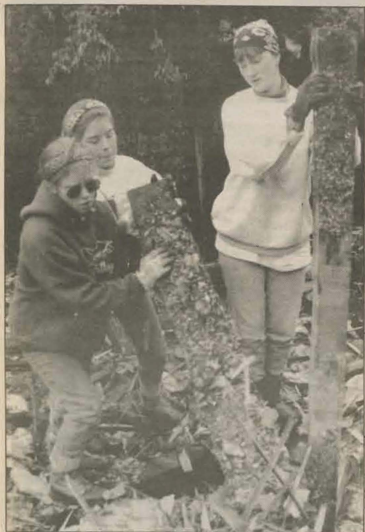
Once the house was demolished by the bulldozer, the remaining debris of glass, wire and nails had to be removed by hand. Erin Burchfield and Heather McDonald pull out one of the fallen rafters while Amy Smith checks for rats.
