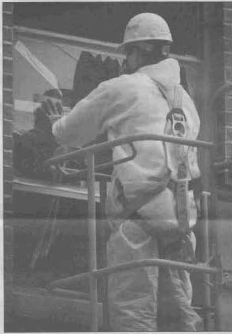
Korsmo Construction Company workers removed glass from windows on the north wing of Eastvold before spring semester began as a part of the renovation.
