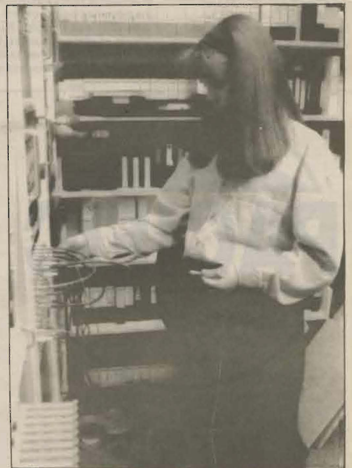
photo by Liz Tunnet Renee Nugent "patches in" audio and visual as part of her training at the KCNS6 control panel.
