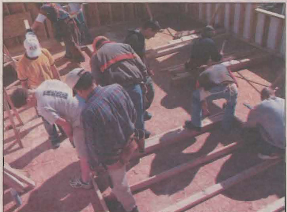
Habitat for Humanity volunteers came together to construct the frame of a house for a family last spring.
