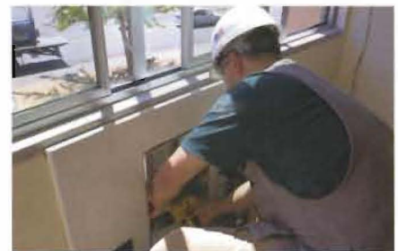
New heating units were installed during the renovation of Pflueger Hall this summer.
