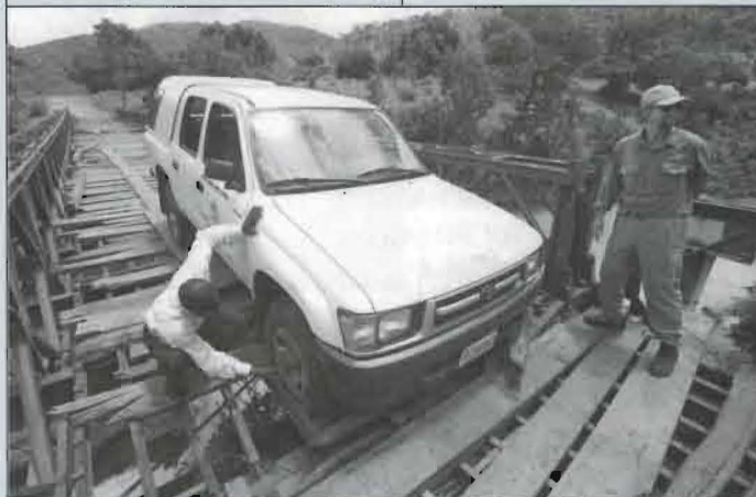
A BRIDGE TOO FAR: Tom Paulson (RIGHT) in Nigeria's central savanna region. While crossing a bridge with driver Inusa Obed (LEFT), the wood planking broke.
