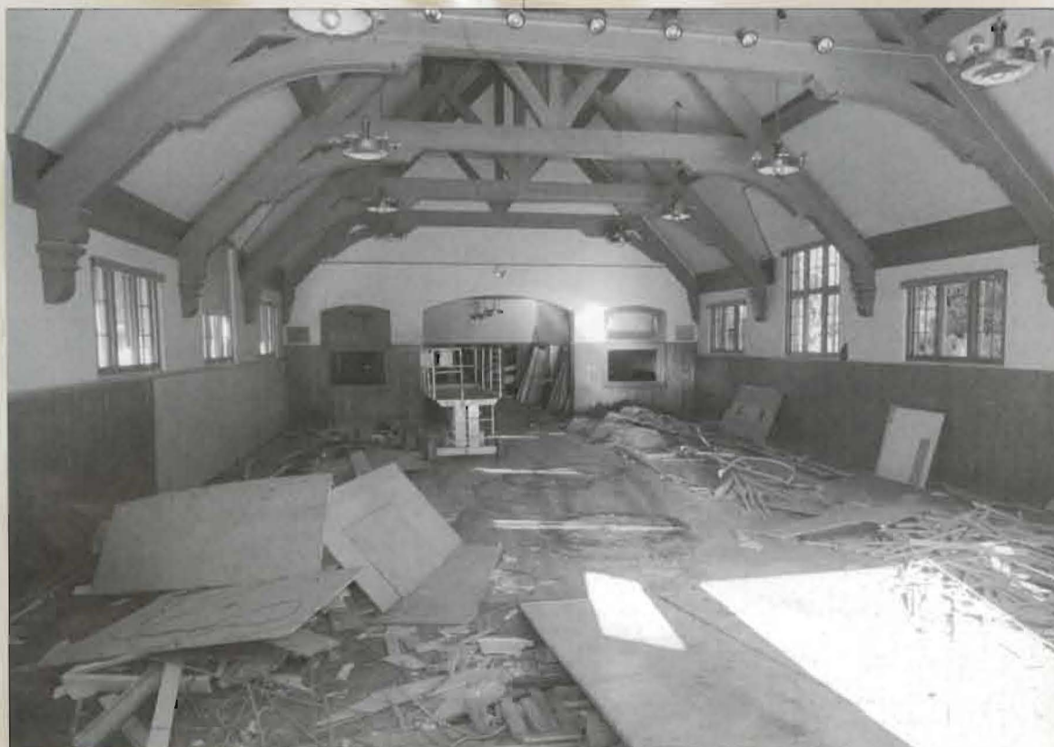
The interior of Xavier Hall is gutted in preparation for extensive remodeling.
