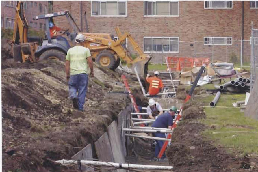
The important work to outfit the campus with the latest technology is all underground.
