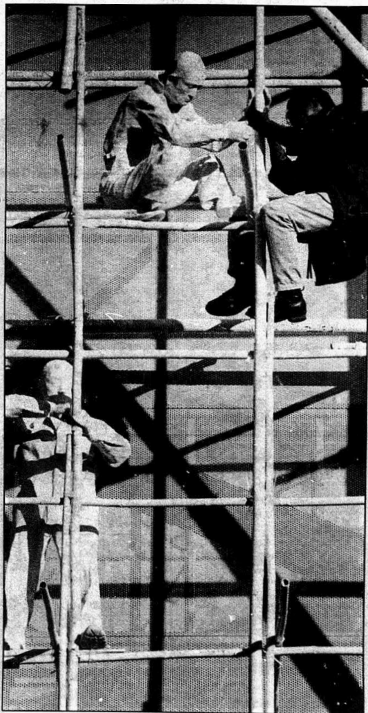
This worker ties plaster mannequins to simulated bamboo scaffolding that envelops the Hong Kong pavilion.
