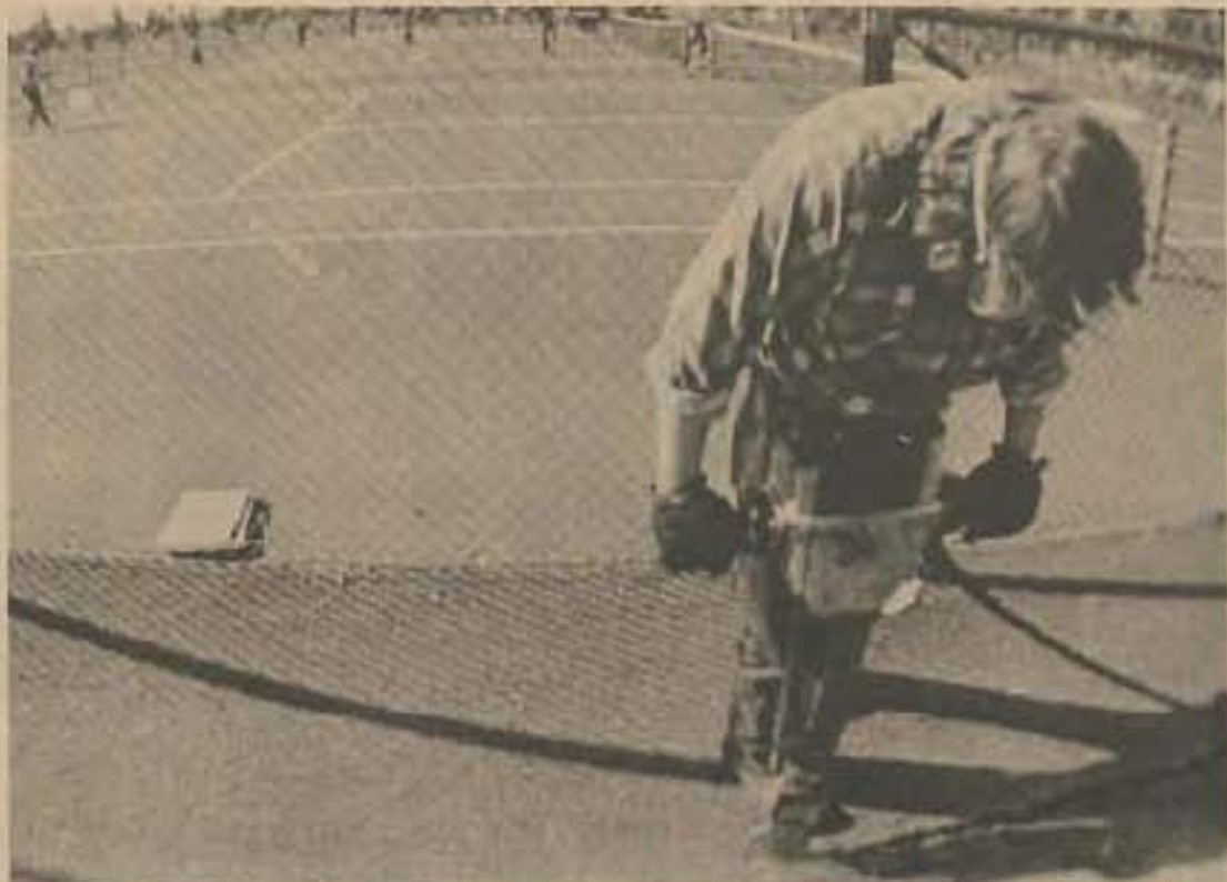
Workman uses jack hammer to prepare ground for new tennis court lights.
